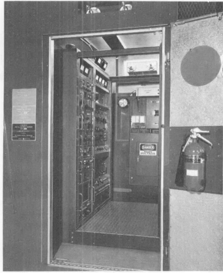
HIGH POWER SHELTER
