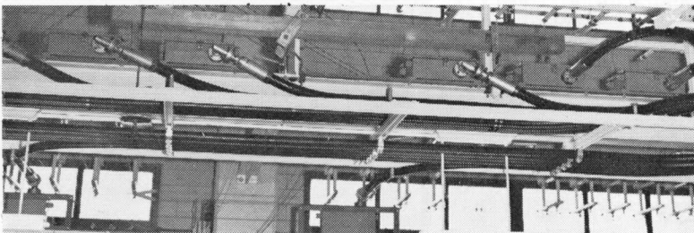
RF POWER distribution cables in a permanent military installation.
