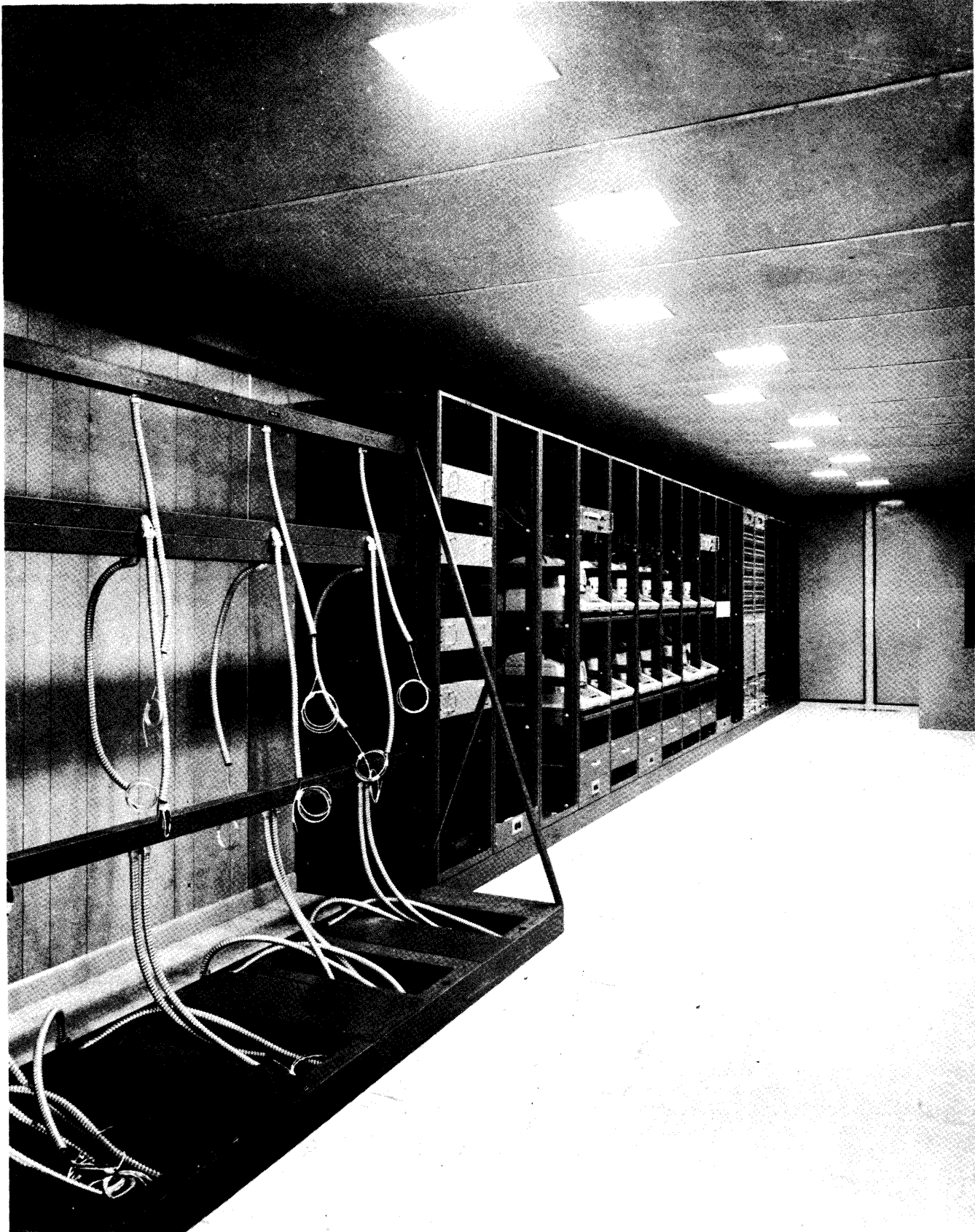
Figure 1-11. Teletype Central AN/TGC-16 (RB1, Equipment Installation)
