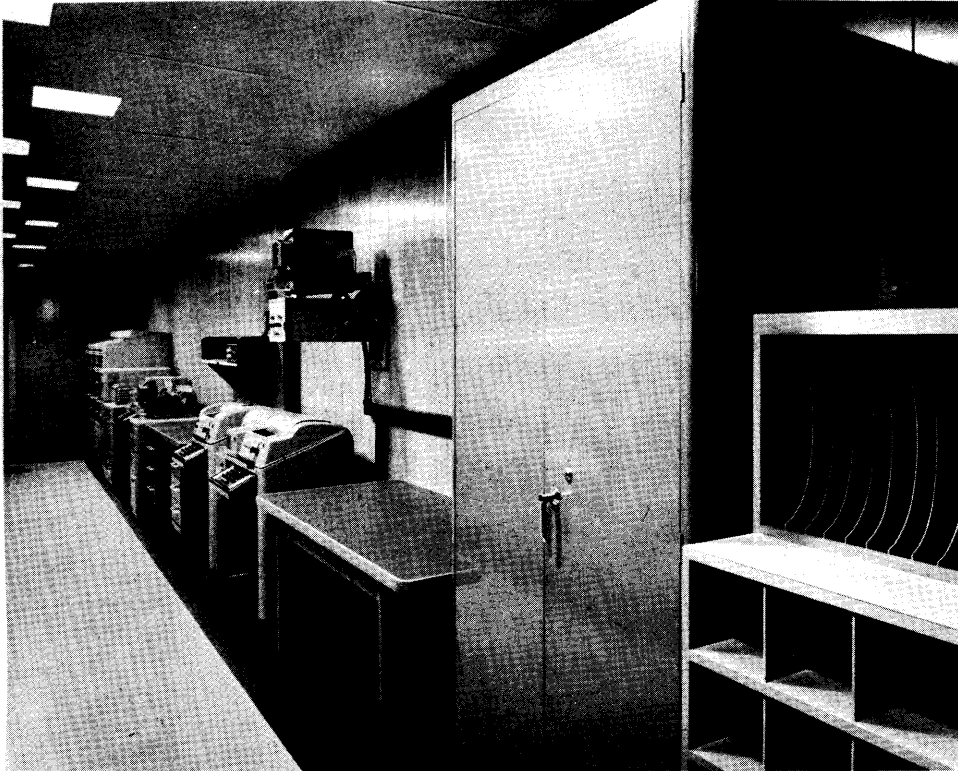
Figure 1-6. Receiving Central Group OA-3887/TSR-1 (RA1 Left Side Equipment)
